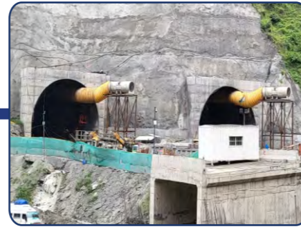
India: NH-44, Ramban Banihal Section (Total Length - 15.976Km) Scope: Feasibility Study, Detailed Design & Construction Supervision
