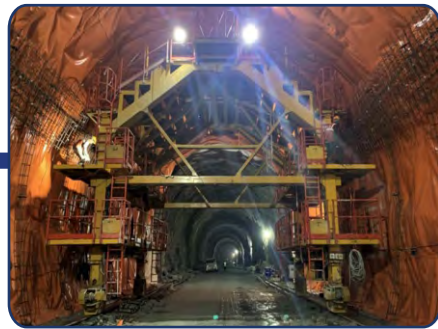
India: Z-Morh Tunnel (Length - 6.412Km) Single Tube Bi-Directional Scope: Independent Engineer for Construction Supervision
